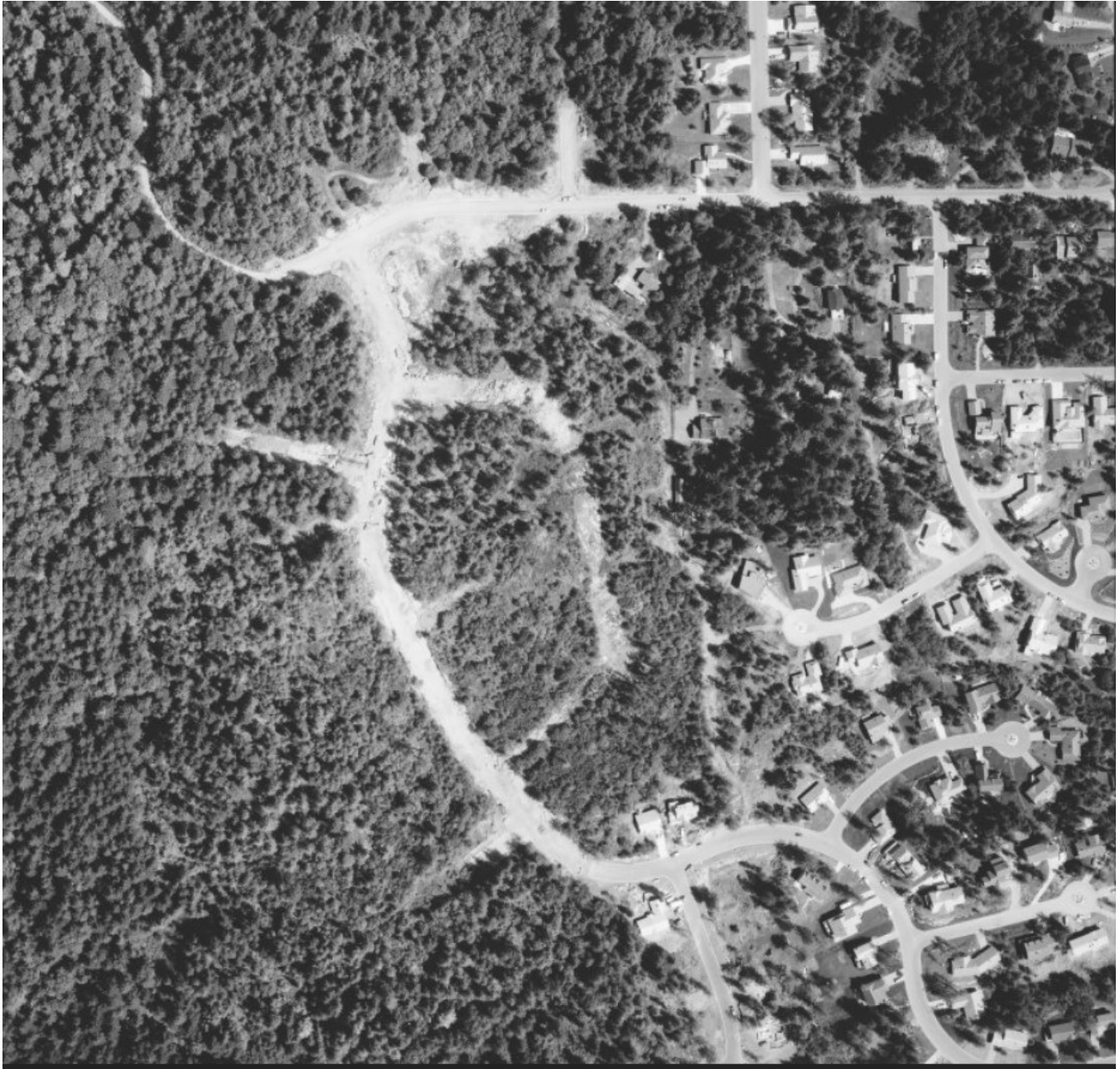
1986 Overhead view of Barrett Drive under construction and Dean Park Road intersection, facing north.
